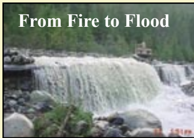
After 8 months without rain, a gully-washer obliterated parts of the North Cascade Highway about 15 miles from Bear Creek Lumber, effectively putting out the fires that had burned all summer. This record rainfall raised river flows by 10 feet in six hours. The highway westbound, seen above, will be closed until sometime next spring.
